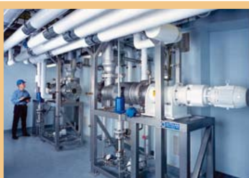
5 sq. ft. Artisan Rototherms® used for solvent recovery at a cGMP facility.
